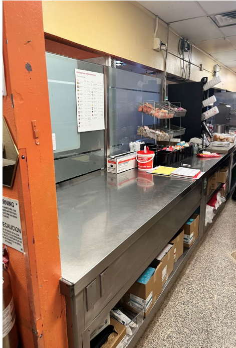
Counter tops and millwork are aged.
