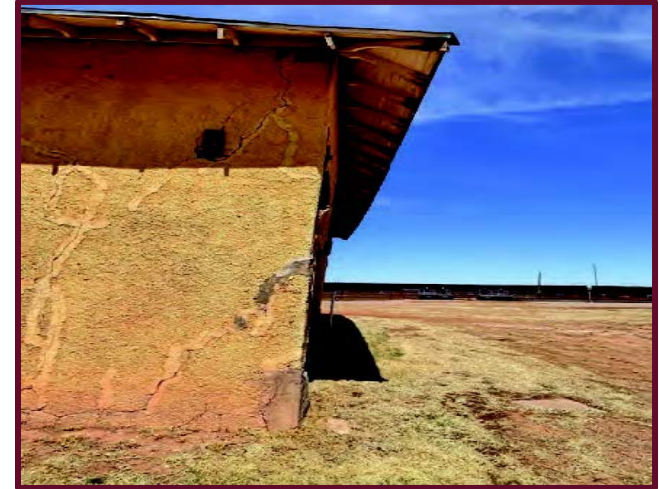
Tucumcari Shop Southeast corner showing wall leaning out with differential settlement
