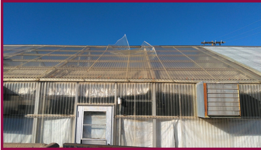
Wind damaged roof panels and ridge cap
