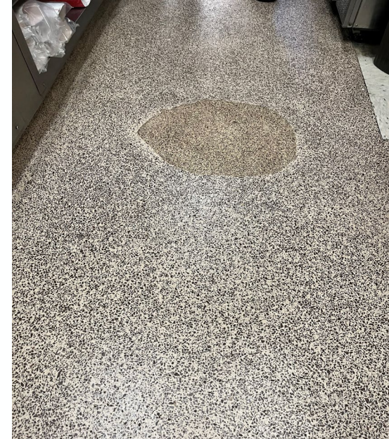
Flooring is aged and becoming more porous. The deterioration of the flooring is a New Mexico Environment Department violation and can be a fire violation as well due to the concrete absorbing grease.
