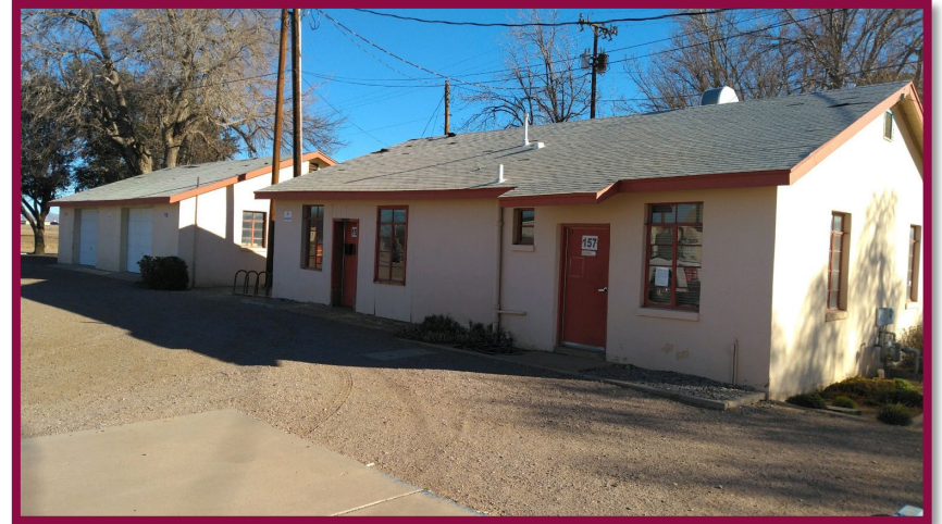
Wind damaged shingles
