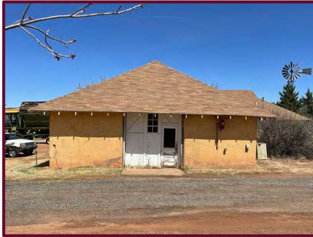
Tucumcari Shop front view showing structural crack and differential settlement
