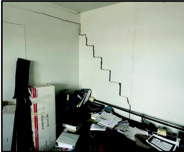
Settlement in interior office
