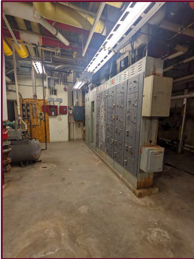
Outdated Electrical Panels
