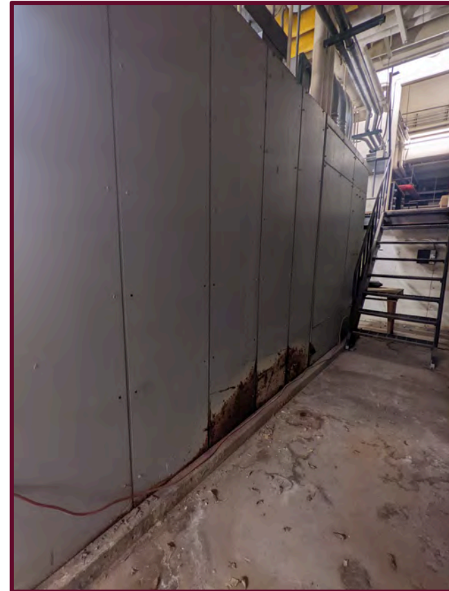
Water damage and corrosion at back of Electrical Panels
