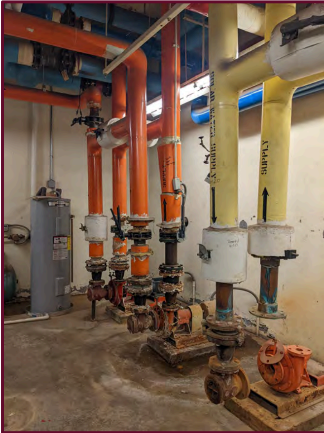
Chilled water utility infrastructure to be removed
