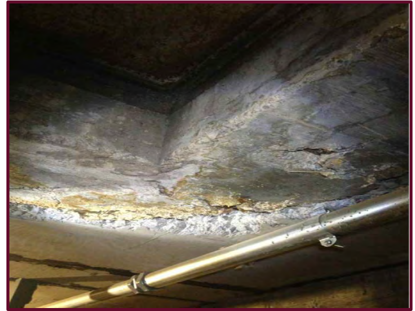
Failing concrete and structural failure of concrete tunnel
