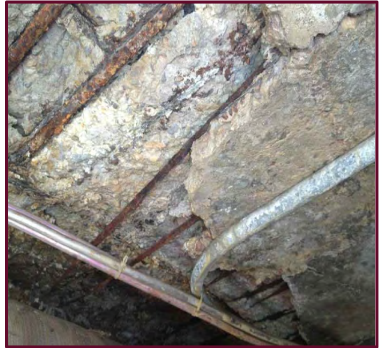
Degradation of Utility Tunnel lid exposed rebar
