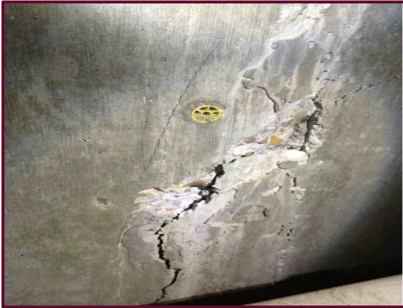
Failing concrete at Utility Tunnel wall
