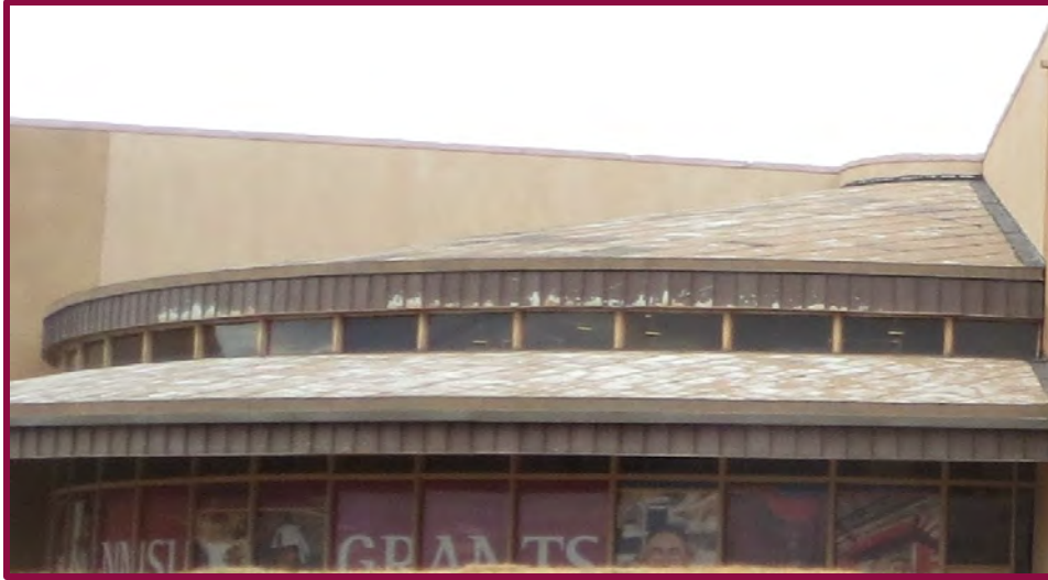
Martinez Hall main entrance roof deterioration view from the entry showing aging roof membrane
