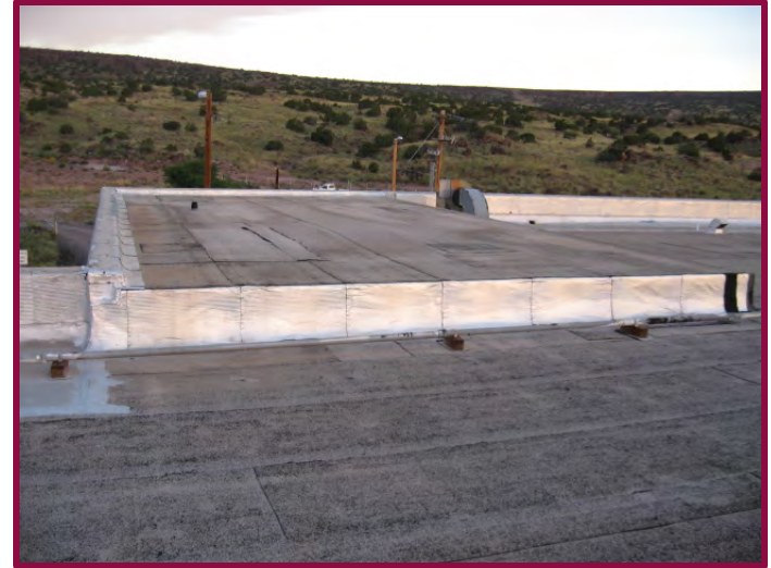
Main roof looking east displaying deteriorating and aged roof membrane
