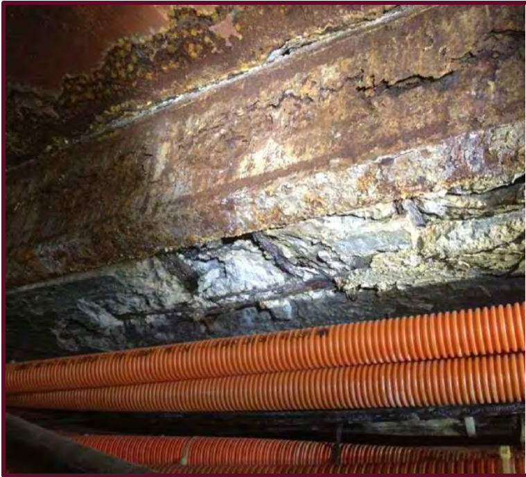
Degradation of Utility Tunnel wall exposed rebar
