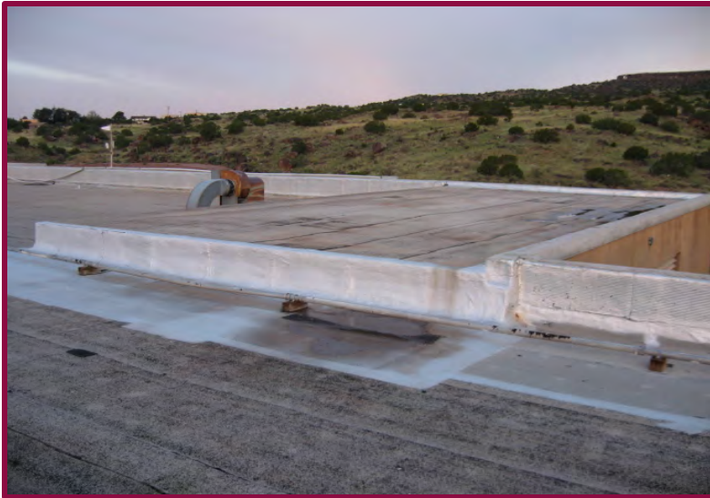
Main roof looking south displaying deteriorating and aged roof membrane
