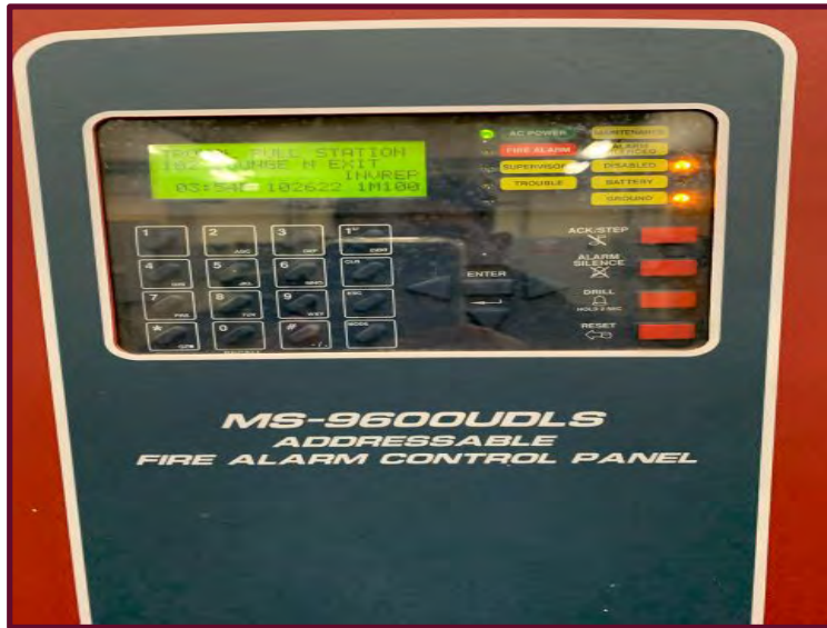
Existing main fire panel
