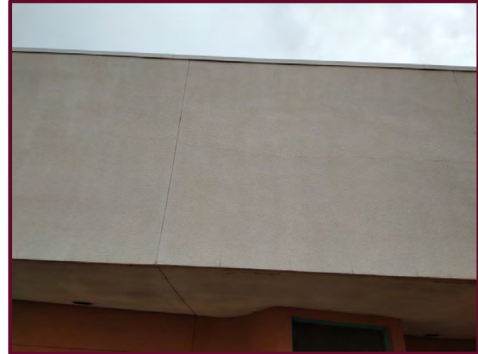
Existing damaged stucco
