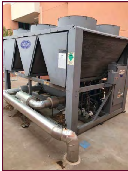
Existing Air Cooled Chiller at west-side, near the Mechanical Room
