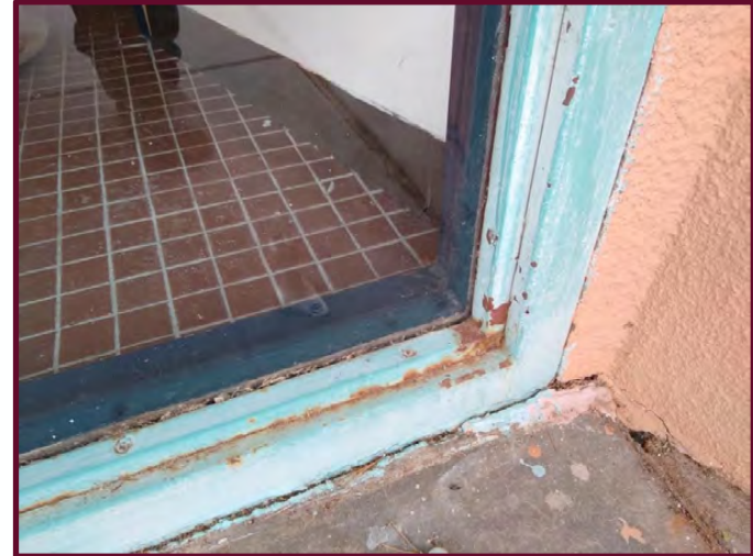
Existing damaged window frames
