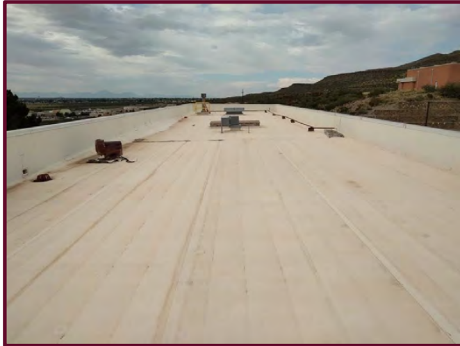
Damaged roofing system
