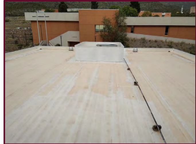
Damaged roofing system
