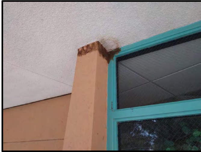
Existing damaged window frames
