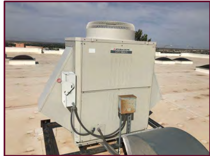
Existing VRF condensing unit on roof
