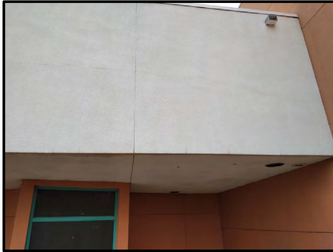
Existing damaged stucco
