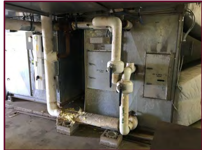
Existing Indoor dual duct unit in Mechanical Room
