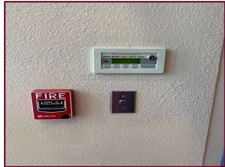
Existing fire alarm pull and controls
