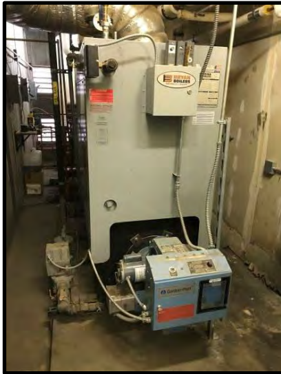
Existing heating HW boiler in Mechanical Room
