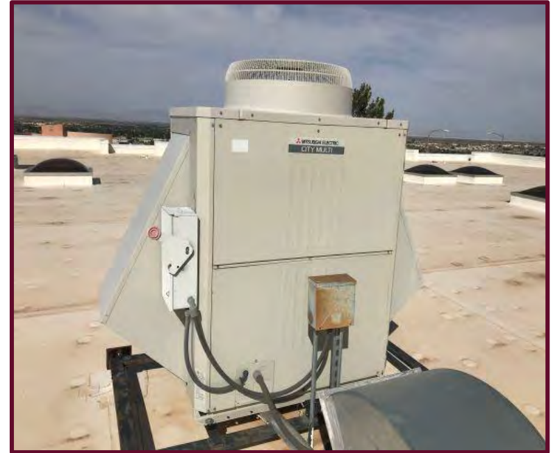
VRF Condensing Unit On Roof
