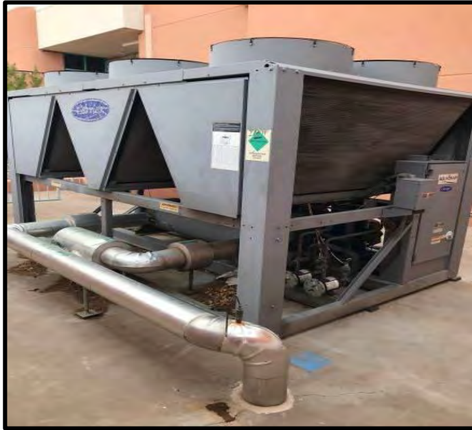
Air Cooled Chiller at West Side of Building
