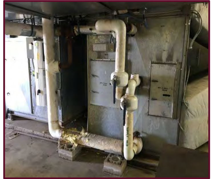
Indoor Dual Duct Unit in Mechanical Room
