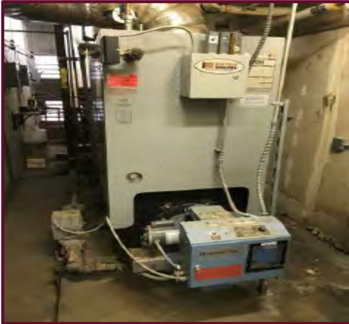
Heating HW Boiler in Mechanical Room
