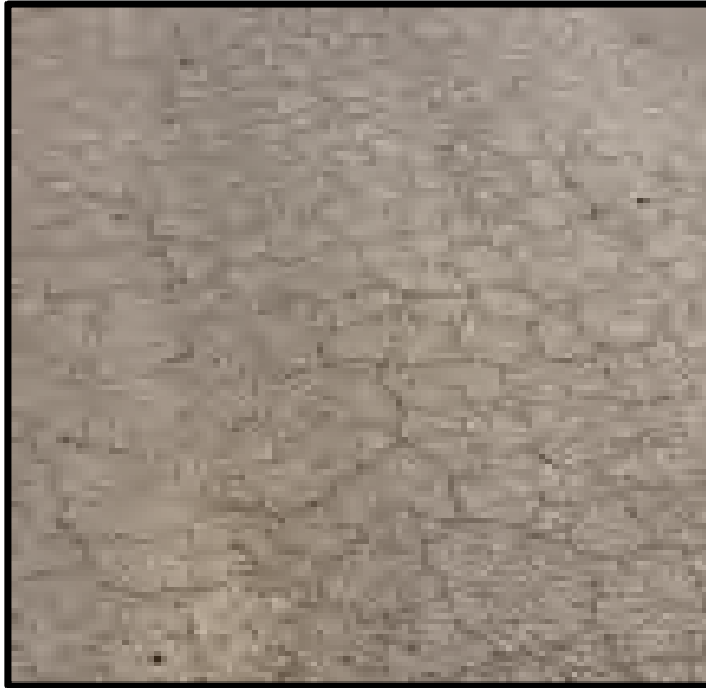
Alligator Cracking where repeated heavy loads or poor subgrade support has cracked the old pavement
