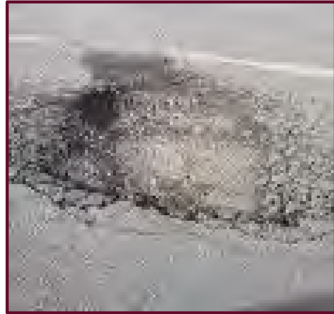
Potholes where pieces of the pavement were lost and moisture collects inside the hole
