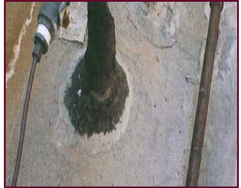
Existing pipe penetration without proper flashing
