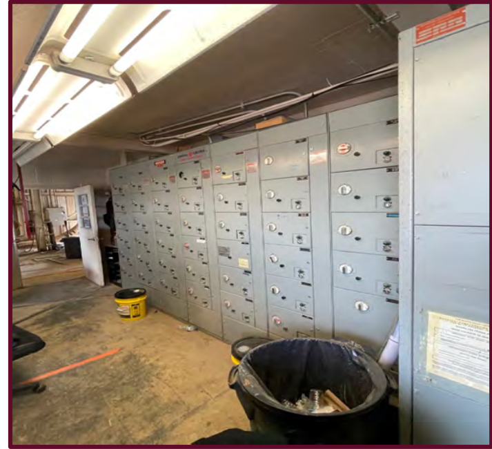
Control Room Electrical Panel
