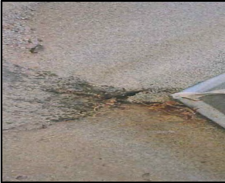
Base flashing to be removed and replaced
