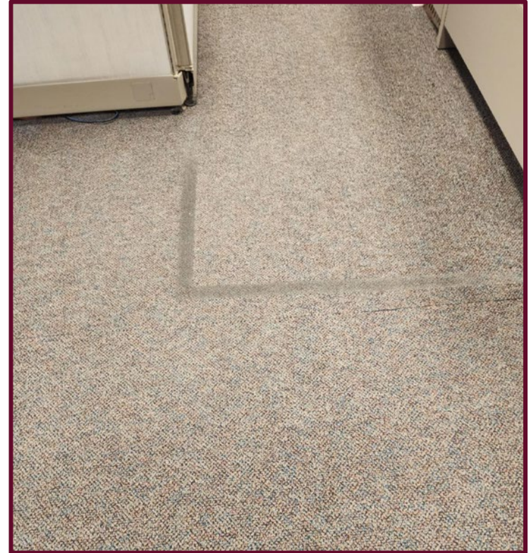
Worn Carpet in Office Space
