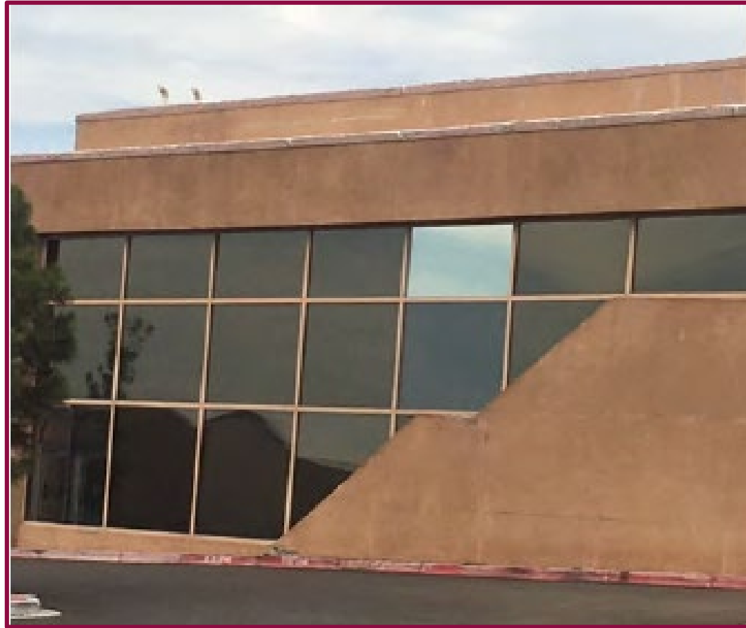
Exterior stucco cracks and deterioration
