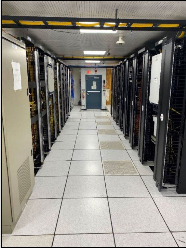
Main data center room
