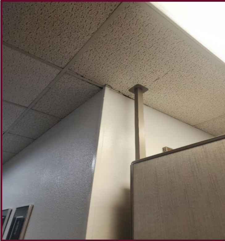
Damaged Ceiling Grid
