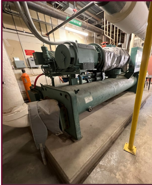
Existing 300 ton chiller out of operation
