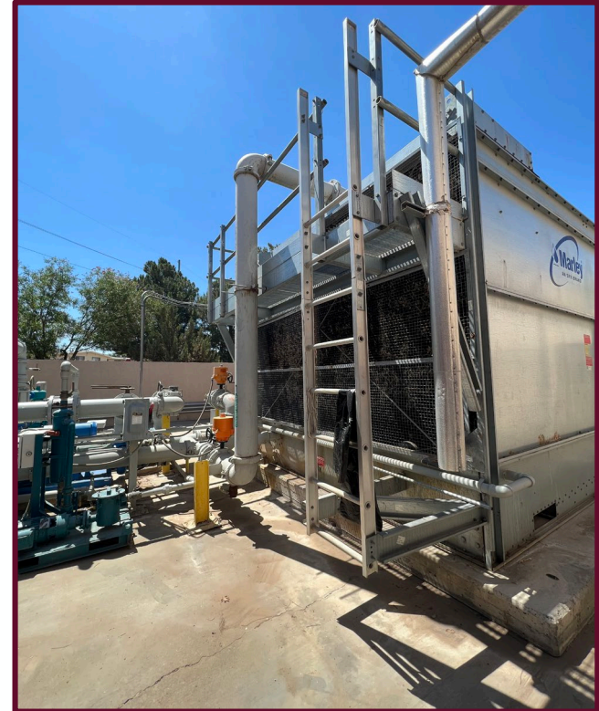
Existing cooling tower and chilled water pumps
