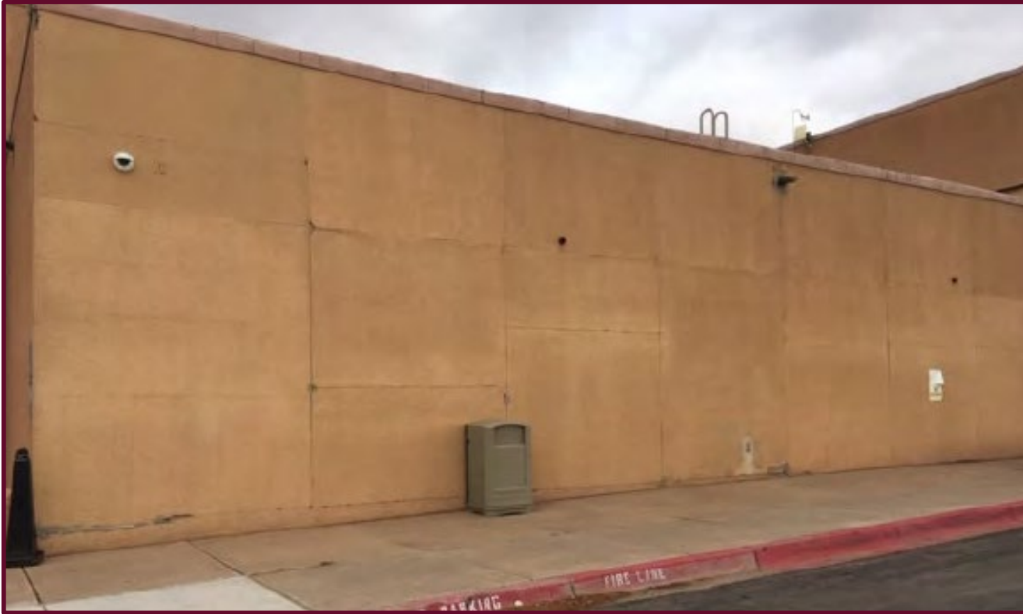
Exterior stucco cracks and deterioration
