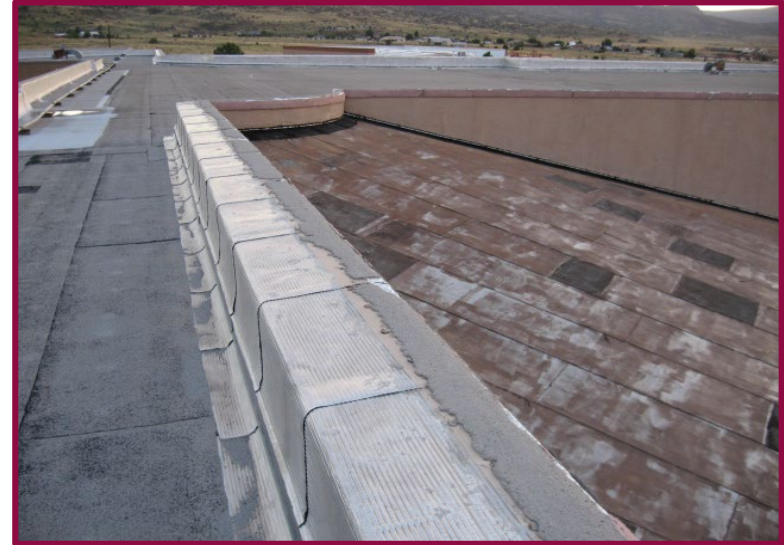
Martinez Hall main entrance view from the top showing roof parapet deterioration and aging roof in need of replacement
