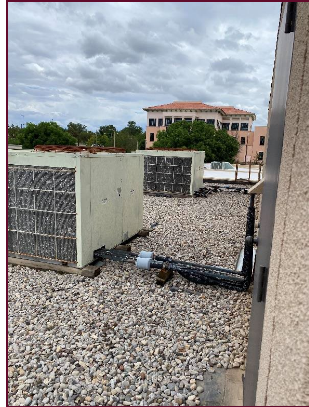
Failed backup condensing units
