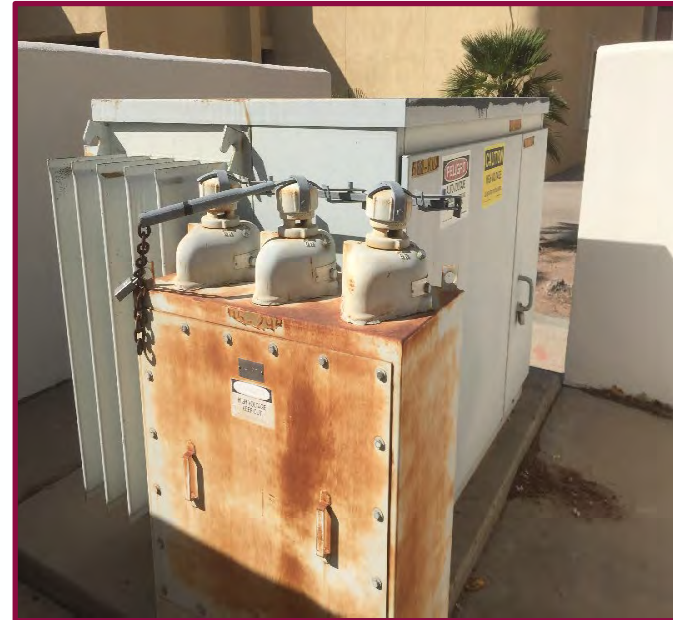
English/Speech 5-kV switch and transformer
