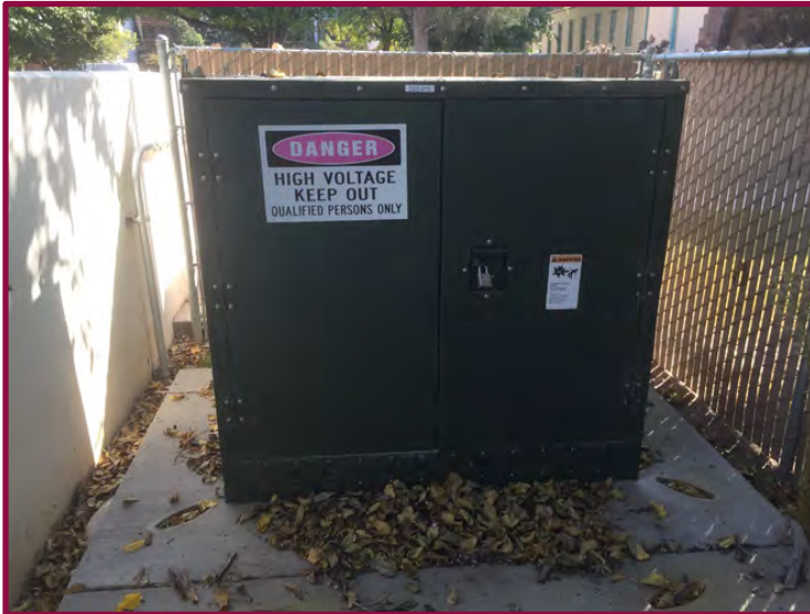
Hadley Hall 25-kV Switch
