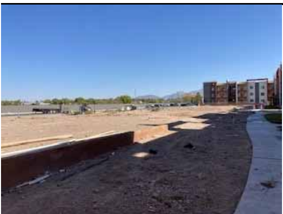
View of the pad sites that will be improved with the two proposed apartment buildings.
