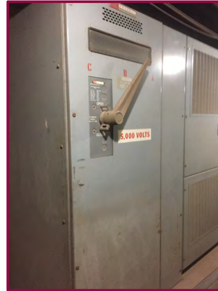
Guthrie Hall 5-kV Switch
