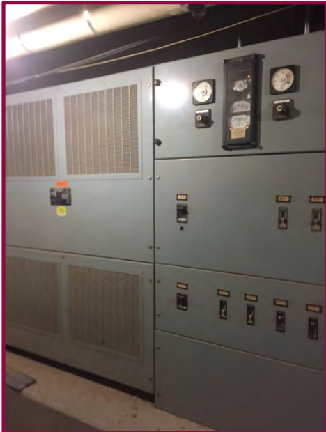
Guthrie Hall Transformer and MDP
