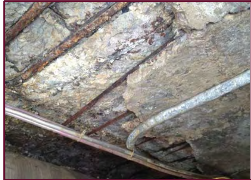
Extensive Reinforcement Corrosion
