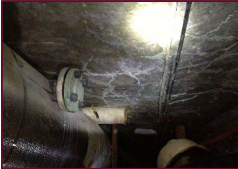
Lid Section Failure
